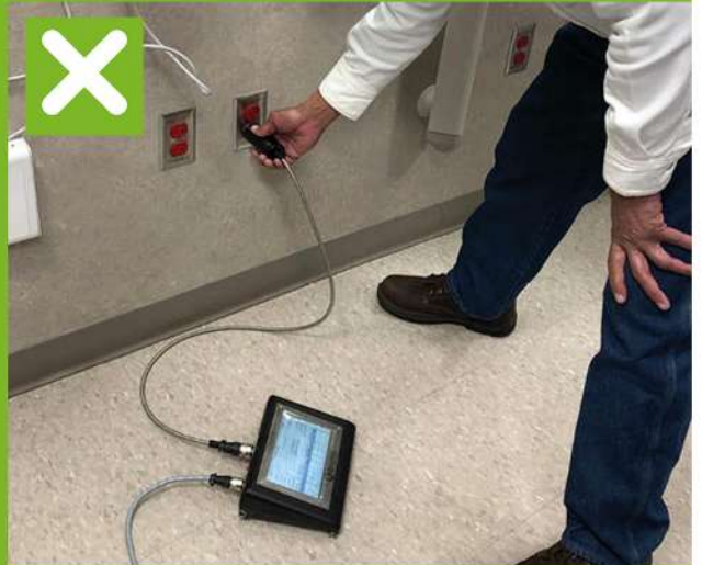
Image: Low electrical port placement in hospital. Ideally points should be 500mm above floor level.
